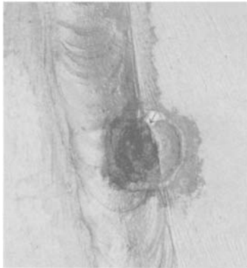
Figure 4.18. Photographs of the corrosion points in tritium installations observed during maintenance or in dismantling. Plate 5: pitting corrosion along the heat-affected zone/fusion boundary of the weld (arrow).
